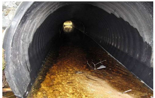
A culvert installed to stream smart principles that is accumulating substrate in the bottom
